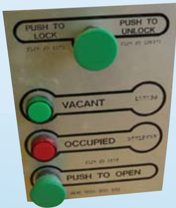
Internal push button control panel with illuminated lights
